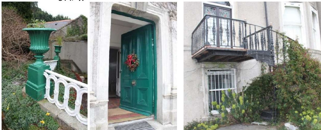
Fig.15.12: Cast iron railing & urn (L), Entrance Door (M), modern steel stair to rear elevation (R)
